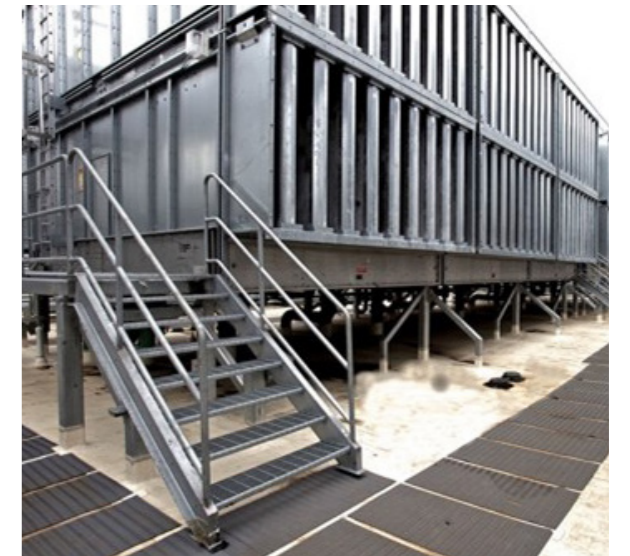
Orlando Utilities Commission Events Center Energy Plant
